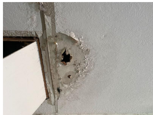
Interior Garage West drywall ceiling Visible water damage Visible microbial growth (>10 sq ft)
