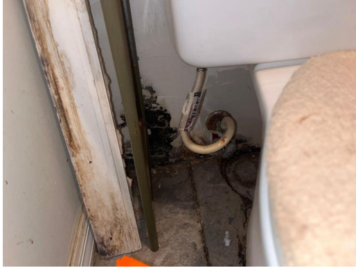
Interior Master Bathroom West lower drywall, wood baseboard Visible water damage Visible microbial growth (>10 sq ft)
