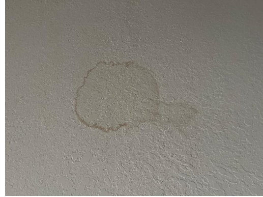
Interior Master Bedroom West drywall ceiling Visible water damage
