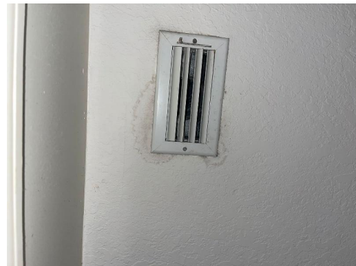
Interior Hall Bathroom West drywall ceiling Visible water damage Visible microbial growth
