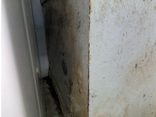
Interior Garage North drywall wall Visible water damage Visible microbial growth (>10 sq ft)
