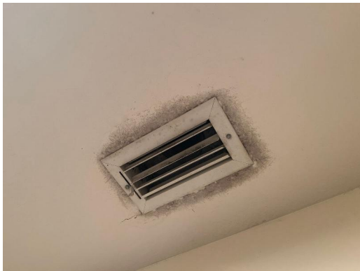
Interior Master Bedroom Drywall ceiling, metal HVAC vent Visible microbial growth
